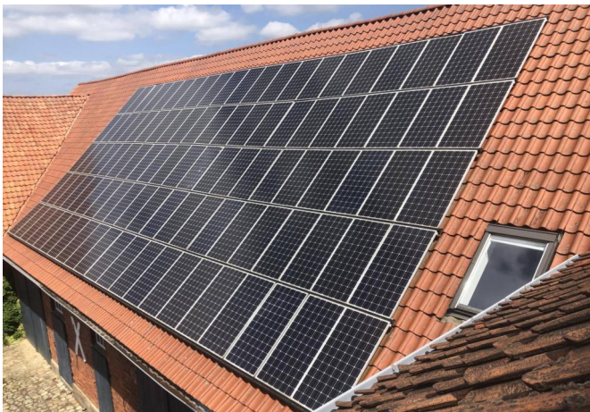
Reithalle - Photovoltaikanlage 19,6 KW/P
